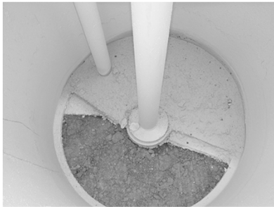
Inside View of Clean out bucket
