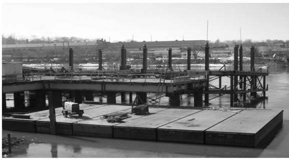
Coffer Dam issues
