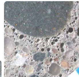
Rating 3 - Severe clustering
