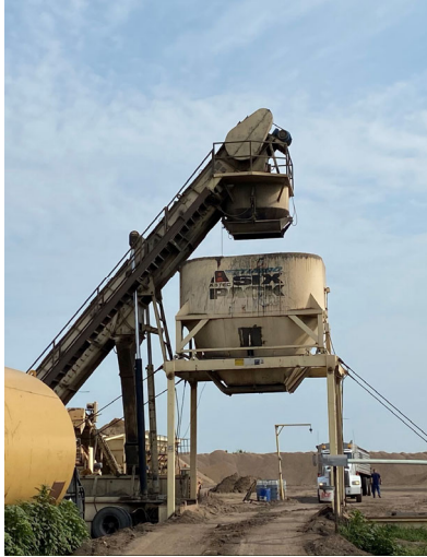
Surge Bin – Net Weight loaded
